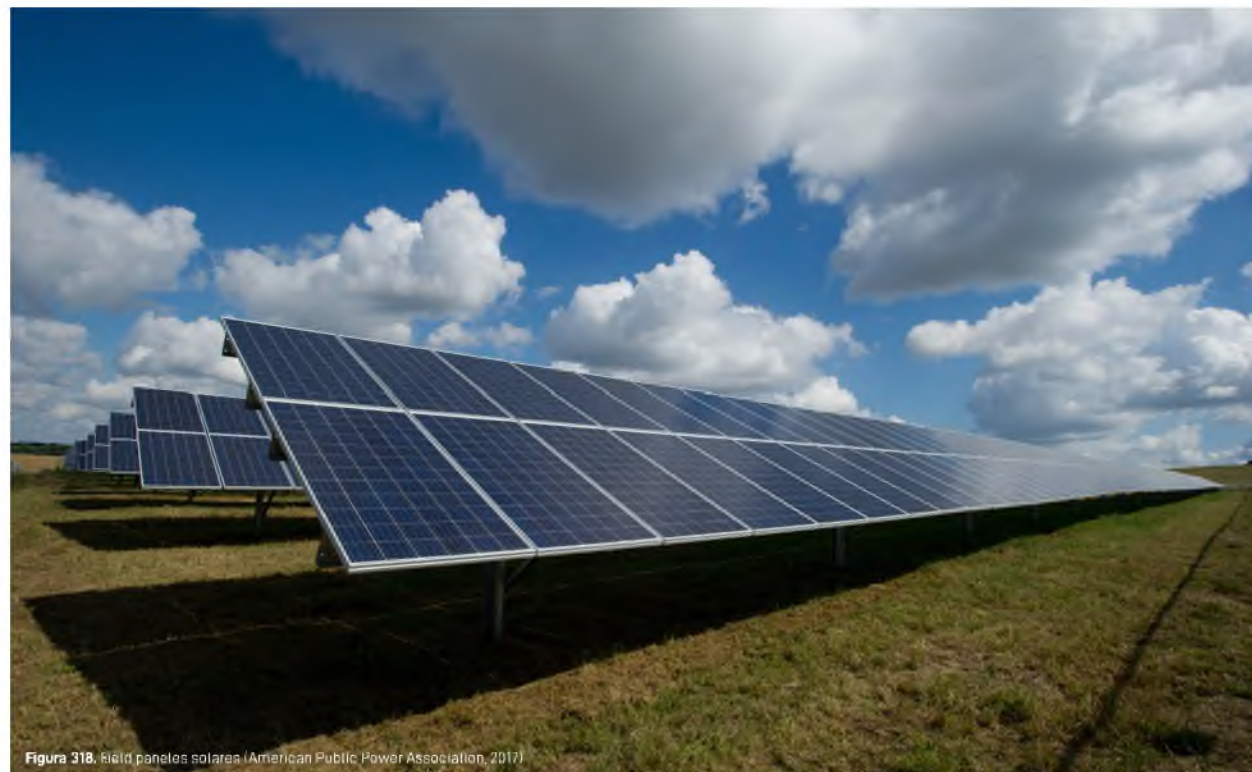
Figura 318. Field paneles solares (American Public Power Association, 2017)
